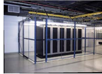
Installed Equipment Racks with Security Enclosure
